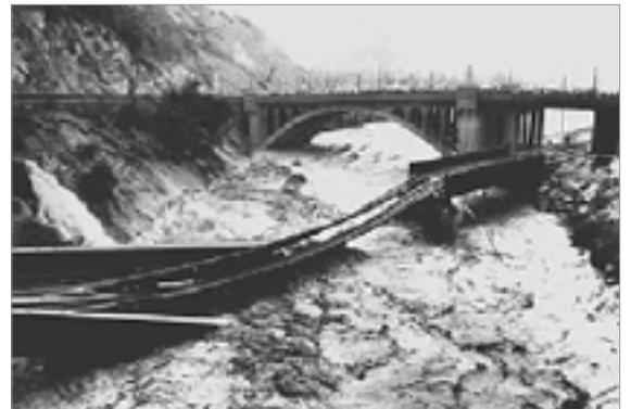
Southern Pacific line damaged in 1938 flood near Figueroa Street in Cypress Park.
