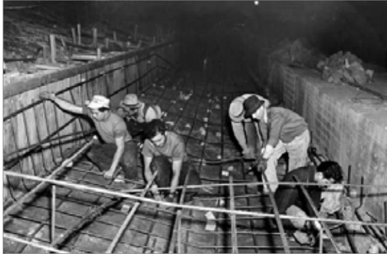
Top: Construction of channel walls at Laurel Canyon in Studio City in the L.A. River by the U.S. Army Corps of Engineers. Courtesy of the Los Angeles Public Library.
